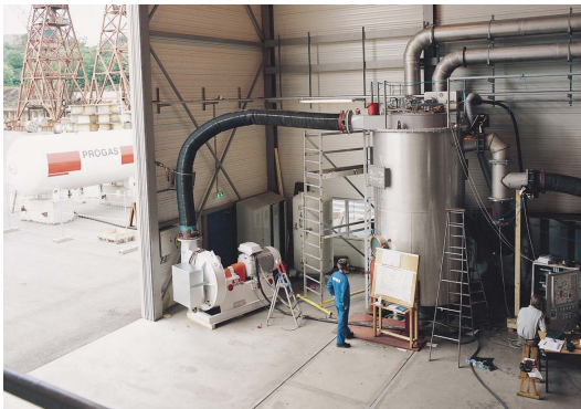
Testing of a dual fuel inert gas generator for a Floating Storage Oil Tanker (FSO). The system comprises 2 generators of 10,000 Nm 3 /h capacity. The generators can burn marine diesel oil or natural gas.
