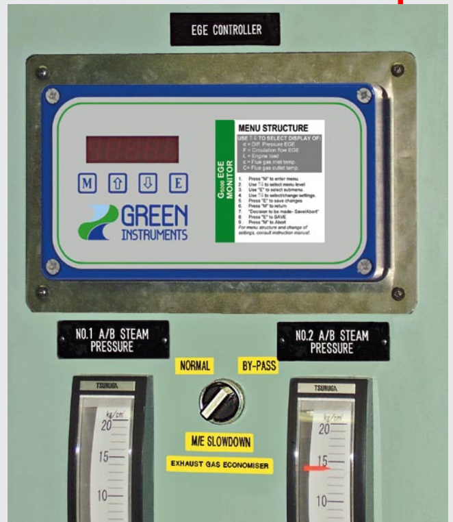
Monitor of the G5000 mounted in a control room panel
